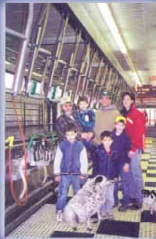
R&R Dairy - Tillamook, OR Parabone Parlor installed by Randy's Dairy Services
