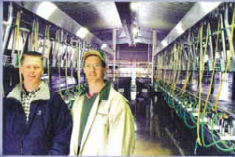
Wavrin Dairy - Mabton, WA Parabone Parlor installed by Excel Dairy Services
