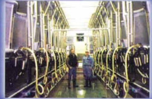
Terral Farms - Yarrow, BC Herringbone Parlor installed by Pacific Dairy Centre
