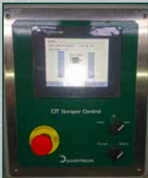
DT Scraper Control PLC Panel
