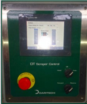
DT Scraper Control PLC Panel
