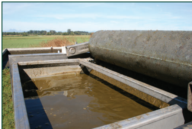
Built in bypass
