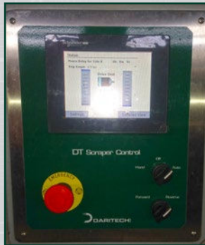
DT Scraper Control PLC Panel
